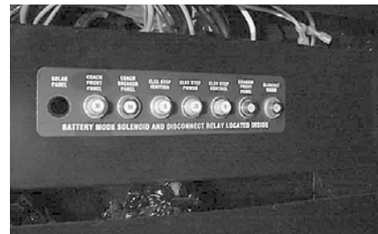
Chassis and House 12V Breakers (cover off)
