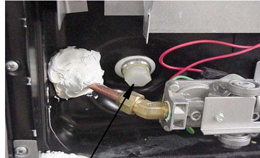
Water Heater Drain Plug Remove with socket
