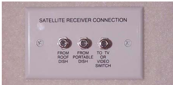
Interior Connection for Satellite Dishes (in front video center cabinet)
