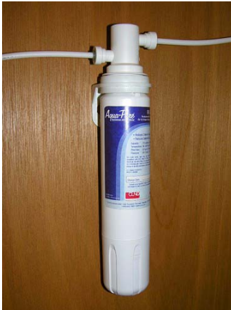
Water Filter Assembly below Galley Sink
