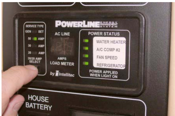
PowerLine EMS Display on Monitor Panel - Typical
