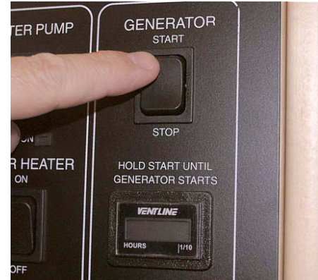
Generator Switch and Hourmeter on monitor panel
