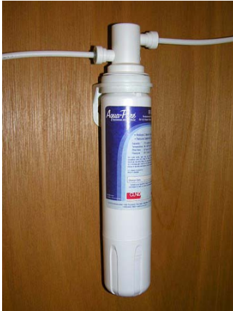
Water Filter Assembly below Galley Sink
