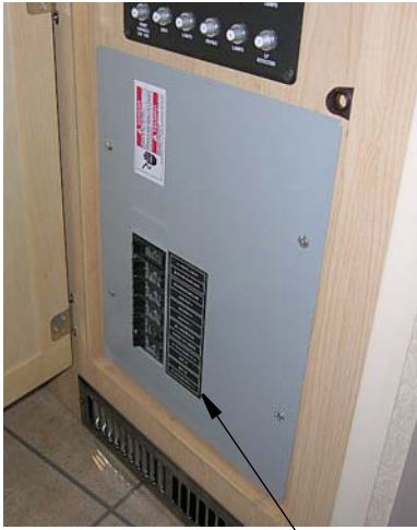
120-Volt House Circuit Breakers - typical
