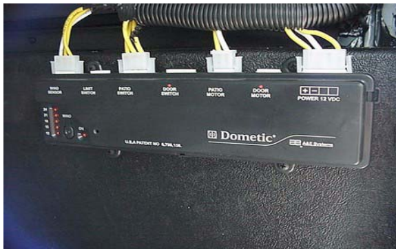
Awning Control Box (located in exterior compartment)
