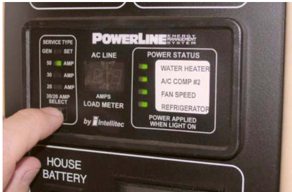
PowerLine EMS Display on Monitor Panel - Typical
