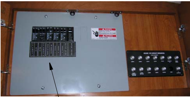
House 120-Volt AC Circuit Breaker Panel
