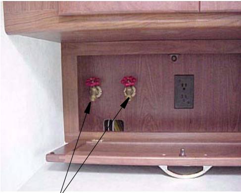
Water Supply Faucets - Typical
