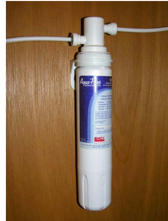
Water Filter Assembly below Galley Sink
