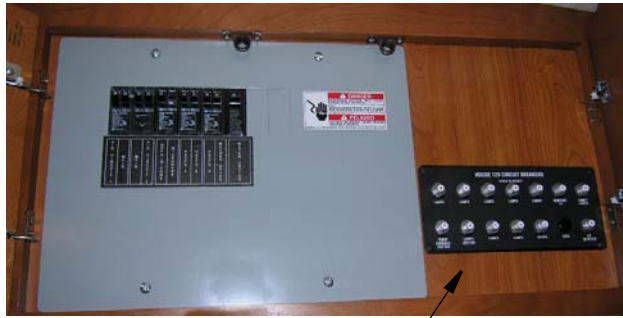
House 12-Volt Circuit Breaker Panel
