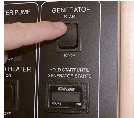
Generator Switch and Hourmeter on monitor panel
