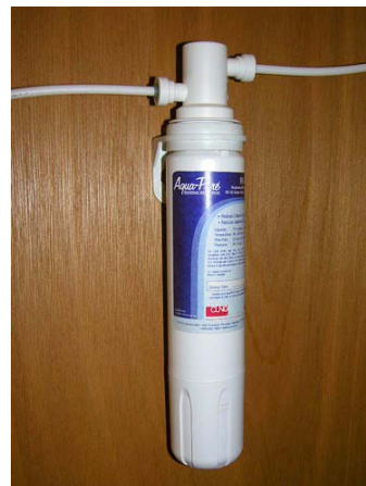
Water Filter Assembly below Galley Sink
