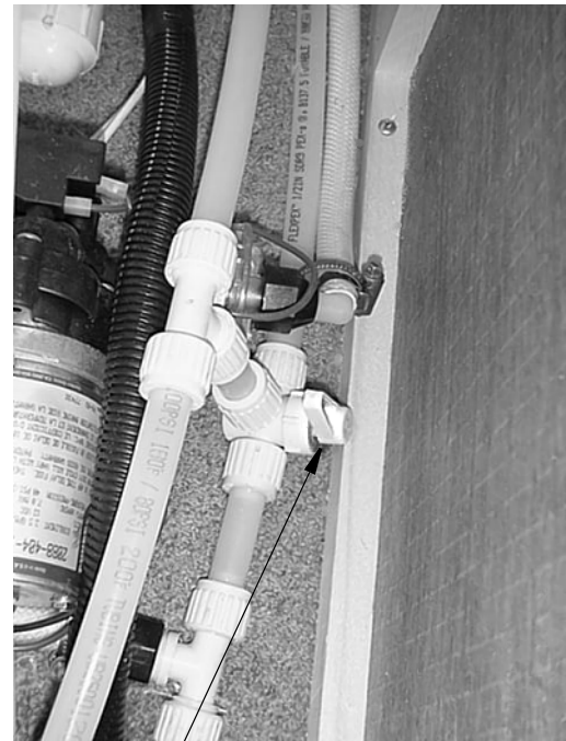
Water Heater Bypass Valve (Typical)
