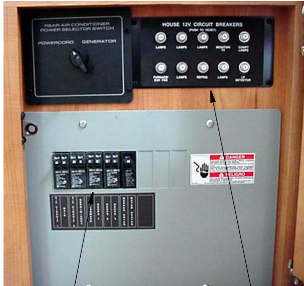
120-Volt House Circuit Breakers
