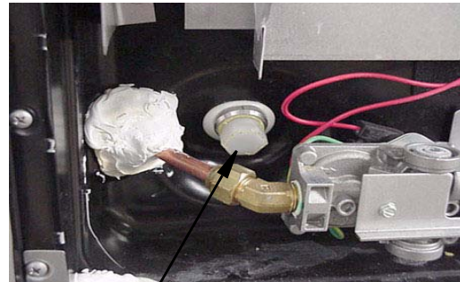
Water Heater Drain Plug Remove with socket.
