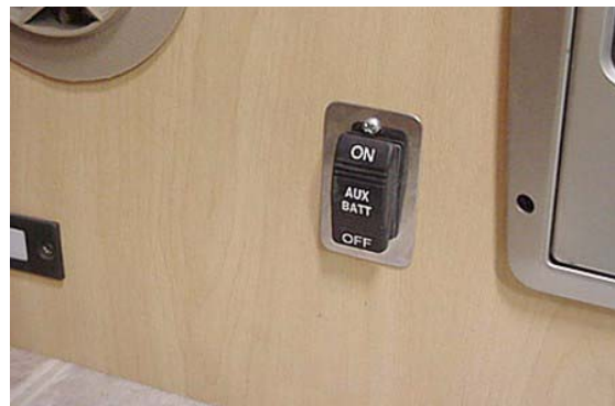
Aux. Batt. Switch - typical (Near entrance door)
