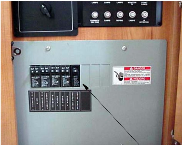
120-Volt House Circuit Breakers
