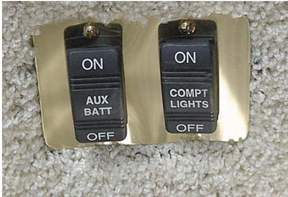
Compartment Lights Switch
