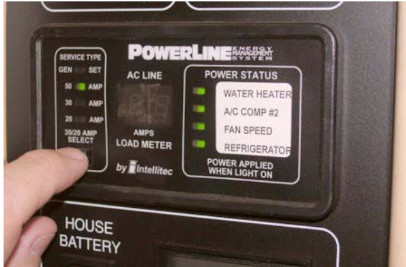
PowerLine EMS Display on Monitor Panel - Typical
