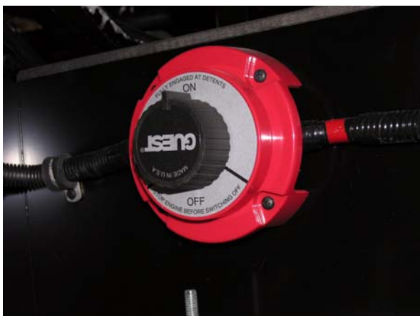
Gas Chassis Battery Cutoff Switch (Inside battery storage compartment)
