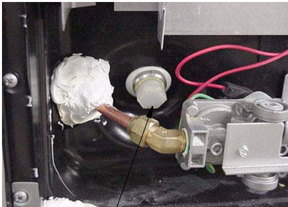
Drain Plug Water Heater Service Access
