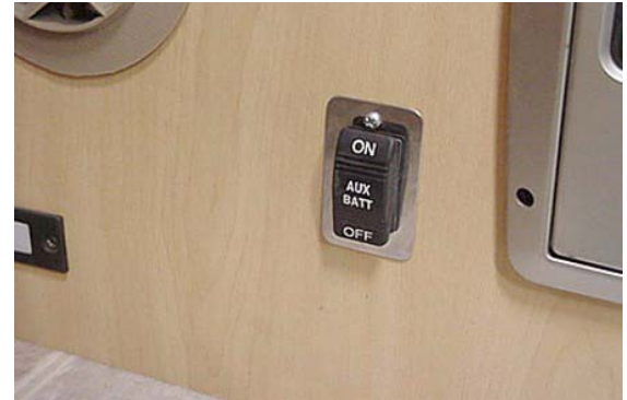
Aux. Batt. Switch - typical (Near entrance door)
