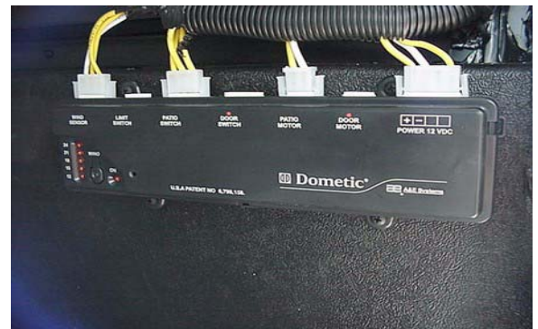
Awning Control Box (located in exterior compartment)
