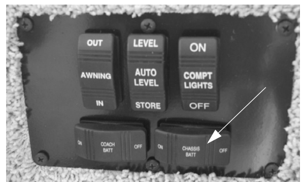
Chassis Battery Disconnect Switch (located inside the entrance door)
