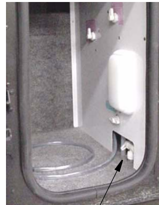
Water Line Drain Valve
