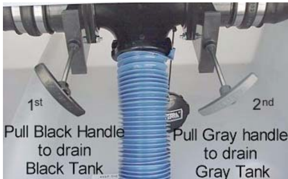
Holding Tank Valves (Typical)
