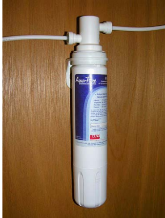
Water Filter Assembly below Galley Sink (Located below galley sink) * Typical View - your coach may vary
