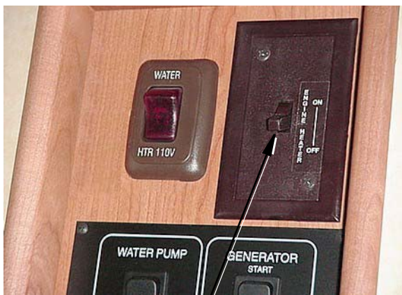
Diesel Engine Heater Switch (typical)
