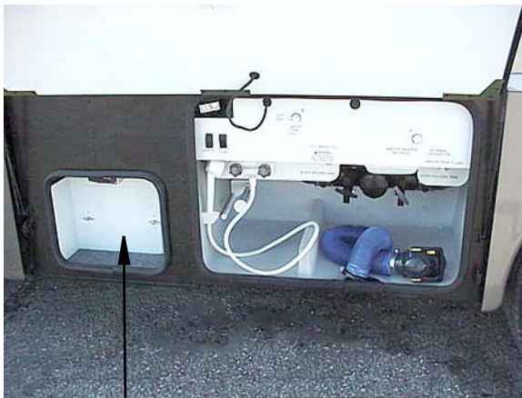
Water drain valves located behind access panel
