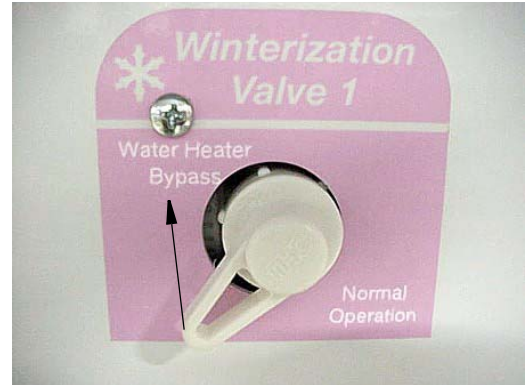
See Water System Drain Valve chart at the end of this section for location on your coach
