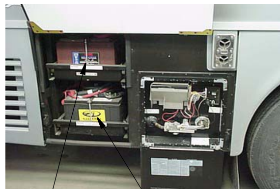
House Batteries Chassis Batteries
