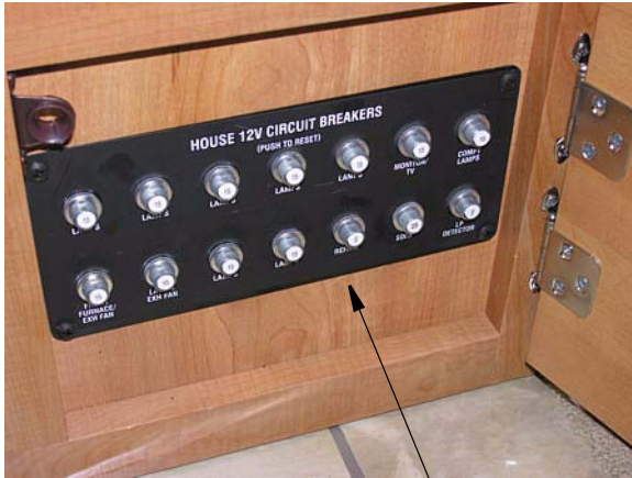
House 12-Volt Circuit Breaker Panel
