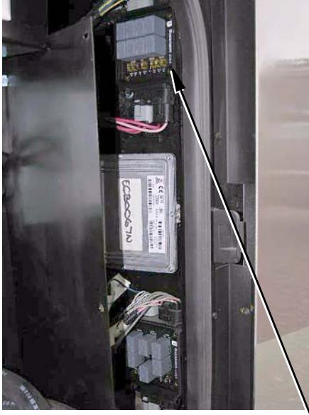
Towing Package fuses are on fuse block
