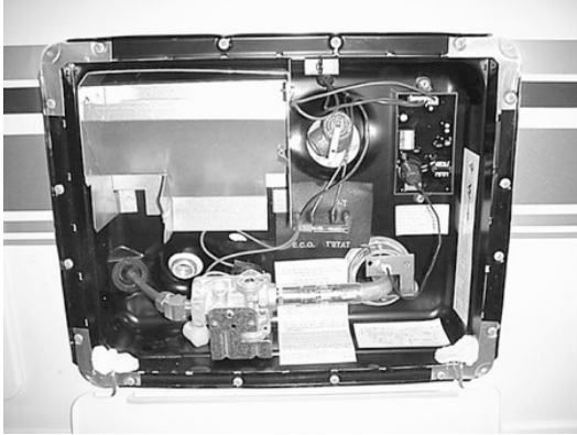
Water Heater Exterior Service Access
