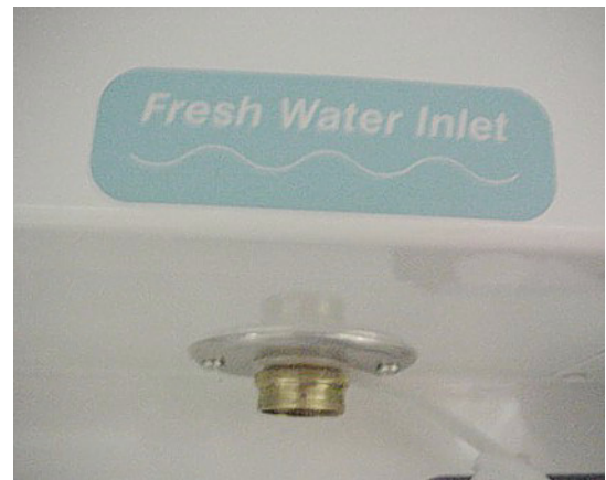
Fresh (City) Water Inlet
