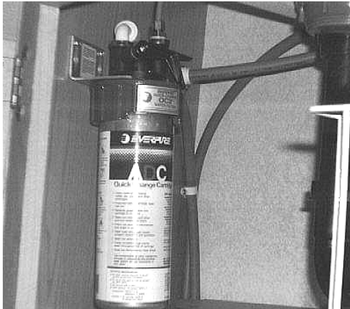
Water Filter Assembly below galley sink
