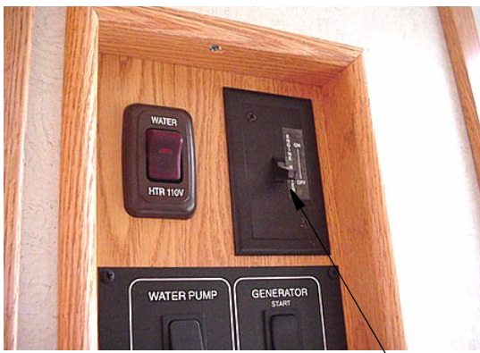
Diesel Engine Heater Switch
