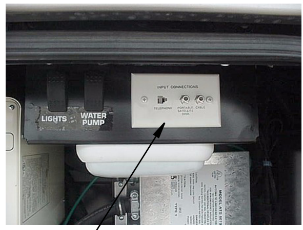
Exterior Input Connections for Satellite Dish, Cable TV and Phone (in Water Center or Shoreline Com-
