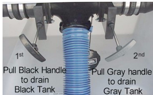
Holding Tank Valves (Typical)
