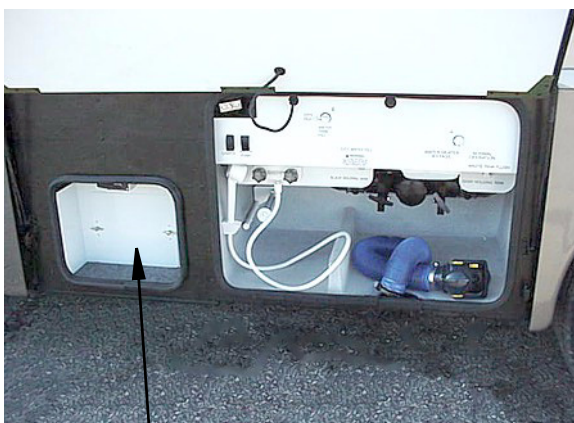
Water drain valves located behind access panel
