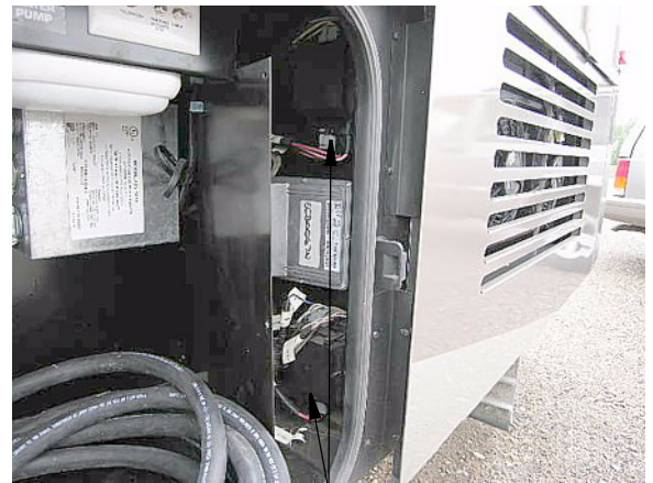
Chassis Fuses and Relays behind close-out panel in Utility Compartment
