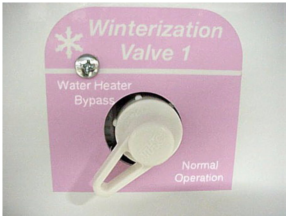
Water Heater By-Pass Valve
