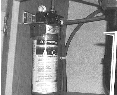
Water Filter Assembly below Galley Sink
