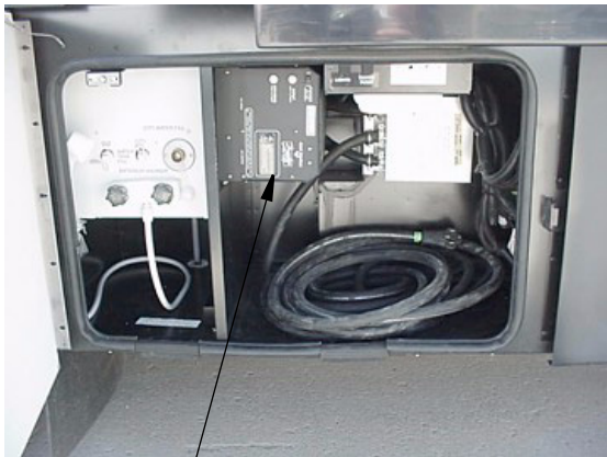
Inverter Charger Unit Location in utility compartment
