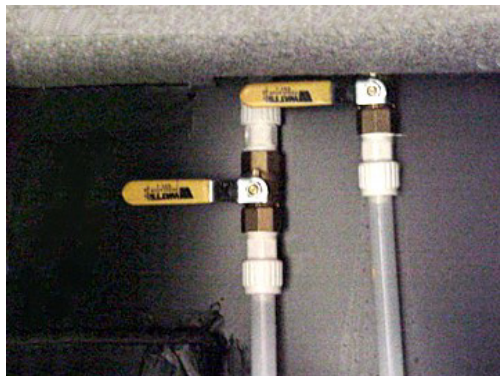
Water Line Drain Valves in Water Center
