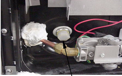
Water Heater Drain Plug Remove with socket.
