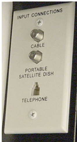
Exterior Connection for Satellite Dishes and Cable TV (In Water Center Compartment)
