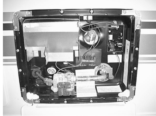
Water Heater Exterior Service Access
