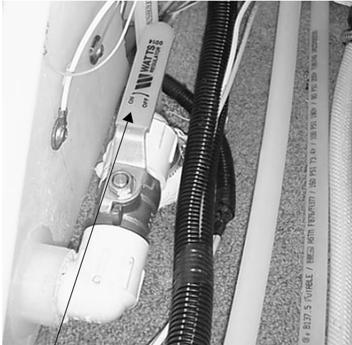
Water Tank Drain Valve
