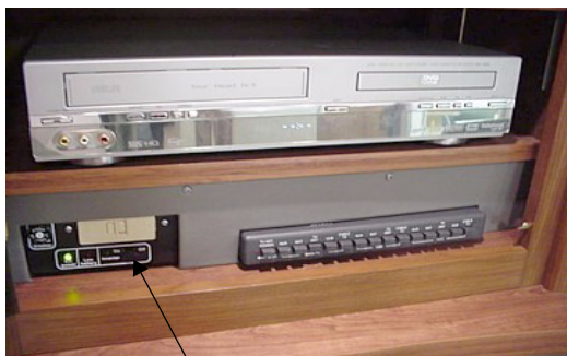
DC-AC Voltage Inverter in Video Center
