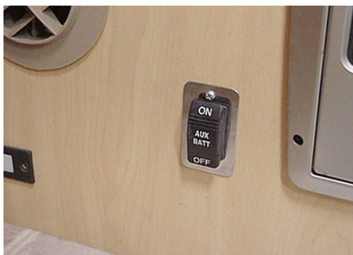
Aux. Batt. Switch (Near entrance door)
