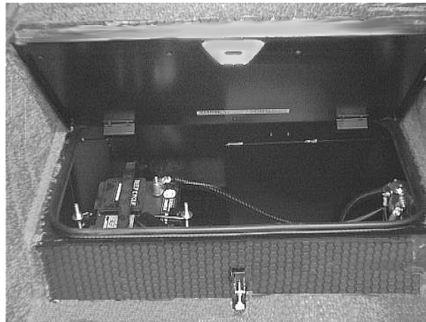
House Battery Storage in Entrance Step
