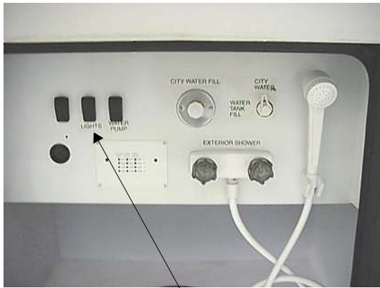
Utility Area Light Switch
