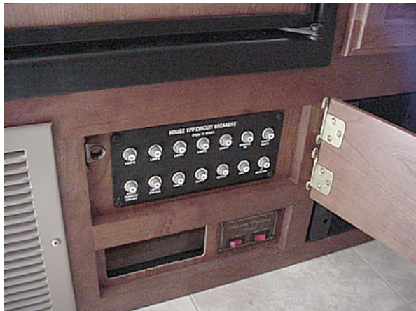
House 12-Volt Breaker Panel
