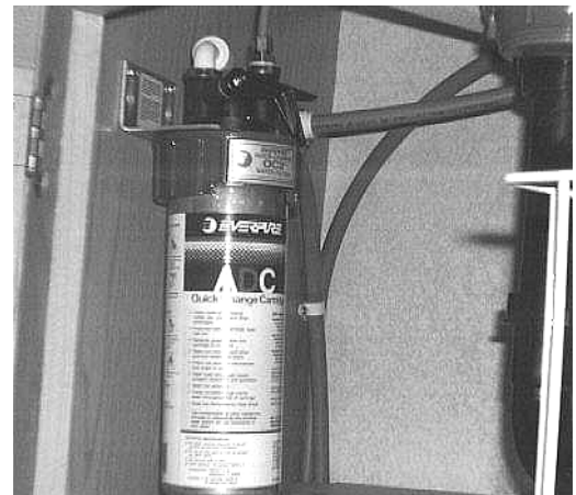
Water Filter Assembly - Below Galley Sink
