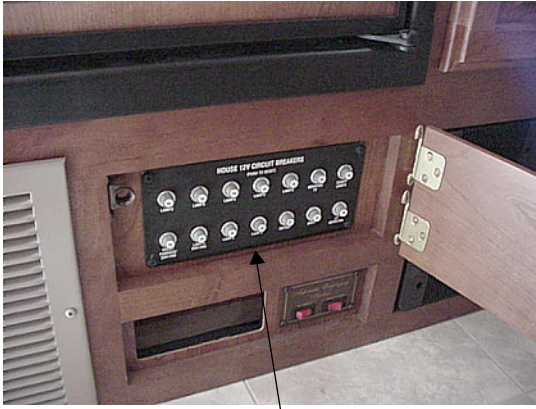
House 12V Breakers
