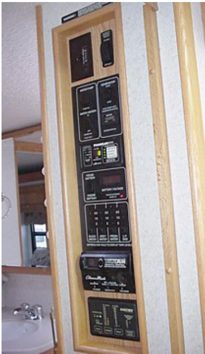
One Place Monitor Panel
