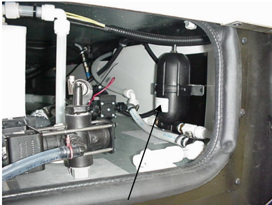
Water Pressure Accumulator Tank
