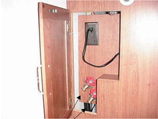
Water Supply Faucets
