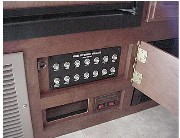
House 12-Volt Breakers
