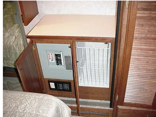
House 110-Volt Breaker Panel in Bedroom Closet
