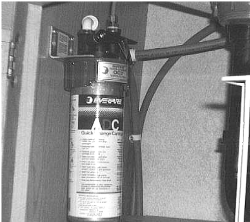
Water Filter Assembly - Below Galley Sink
