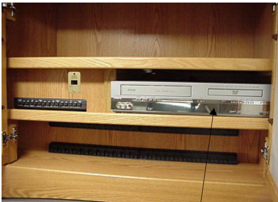
Video Selection System in Entertainment Center Cabinet
