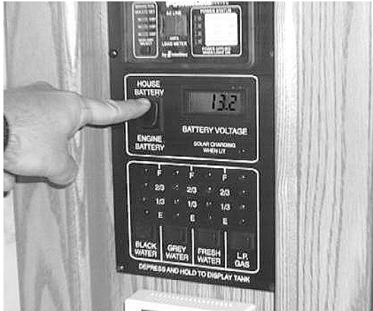
Battery Voltage Check One Place Panel
