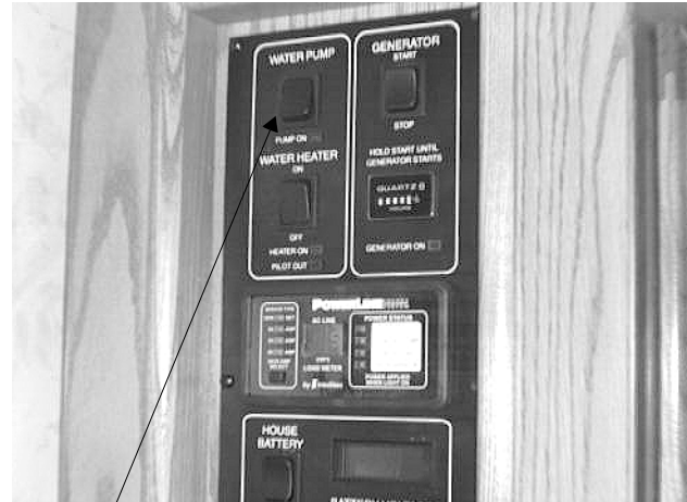
Water Pump Switch
