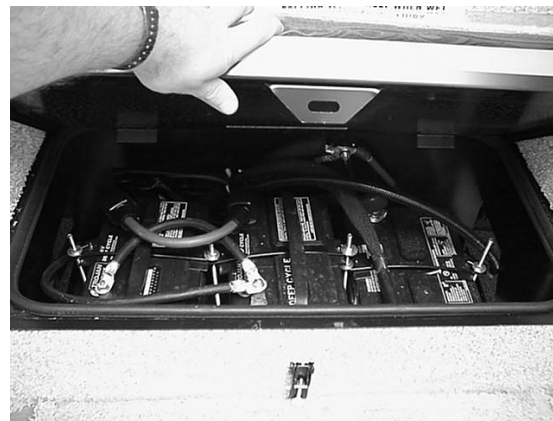
Lift step to access batteries
