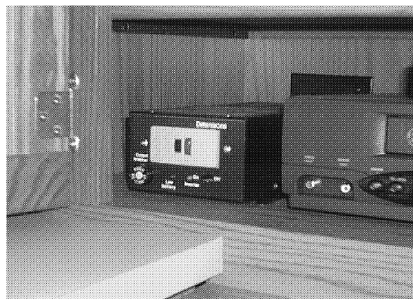
DC-AC Voltage Inverter in Video Center
