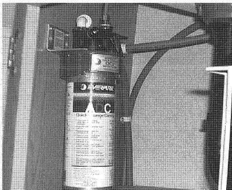
Water Filter Assembly - Below Galley Sink
