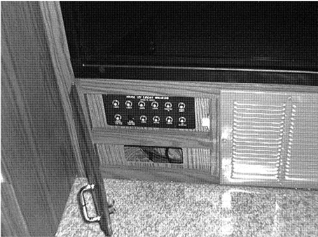
House 12V Breakers (below refrigerator)
