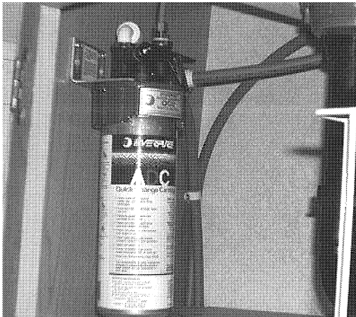
Water Filter Assembly - Below Galley Sink
