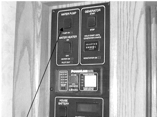
Water Pump Switch
