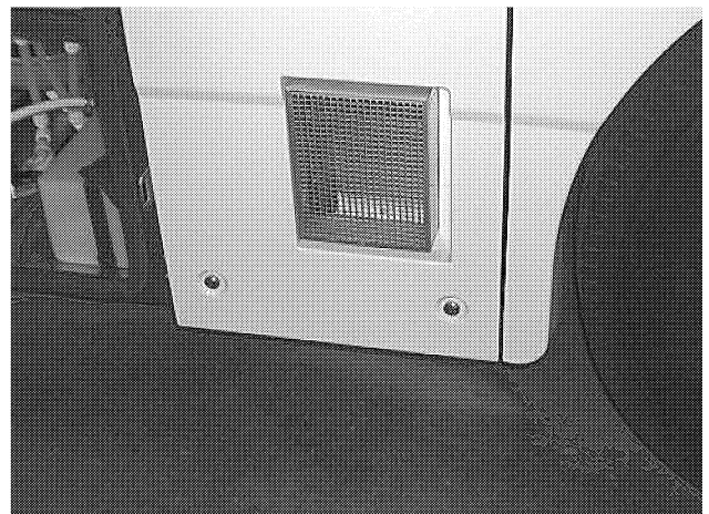
Water Heater Service Access Panel
