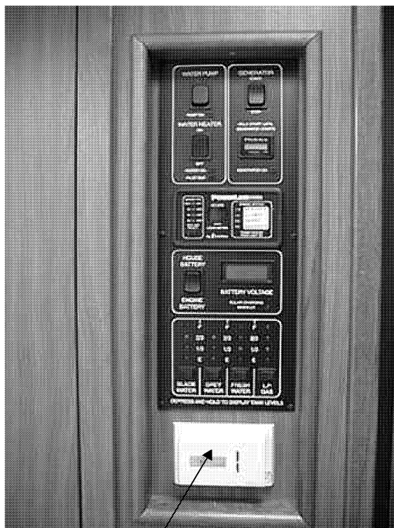
Power Vent Thermostat Bath Area
