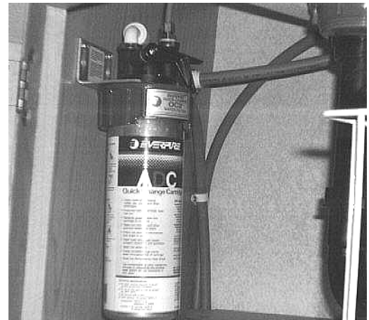
Water Filter Assembly - Below Galley Sink
