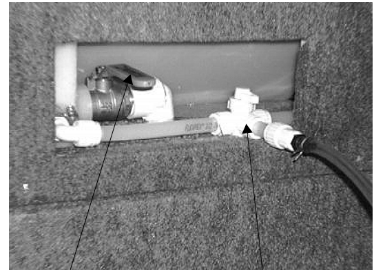
Water Tank Drain Valve
