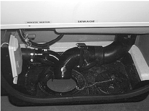
Holding Tank Dump Valves
