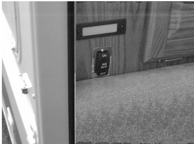
Aux. Batt. Switch (Near entrance door)
