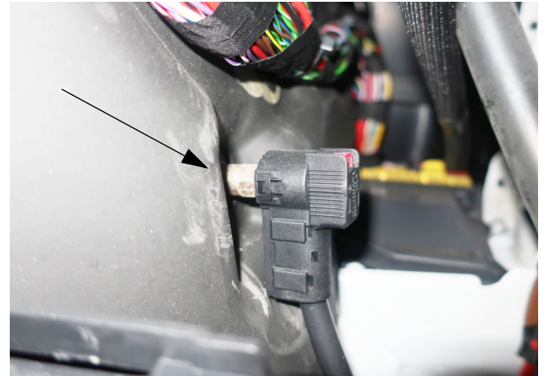
Chassis Battery Connector (Located to the right of the accelerator pedal inside access panel)
