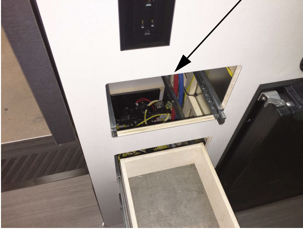
Water Pump (Located below galley cabinet - remove galley drawers to access)
