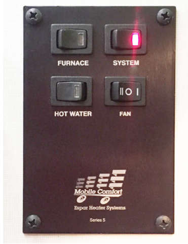
Switch Panel (Located near monitor panel)
