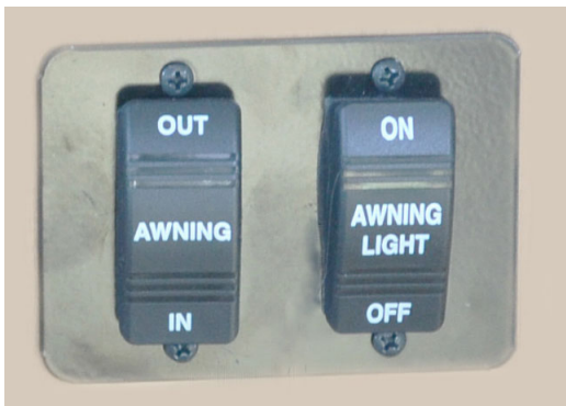
Power Awning Switch and Awning Light Switch (if equipped) (Located at front of galley) -Typical View
