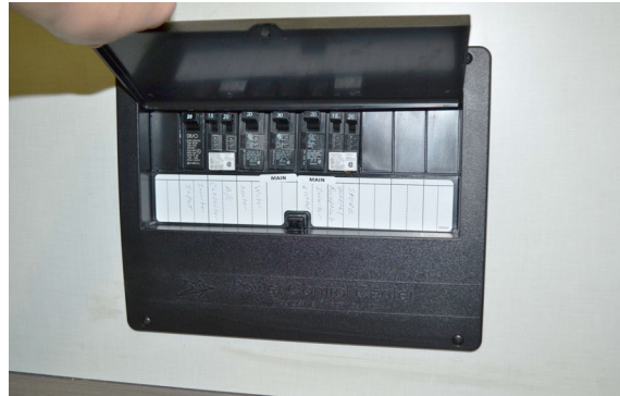
120-Volt Circuit Breakers -Typical View
