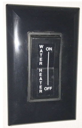
AC Heating Switch (Electric) (Located near monitor panel)
