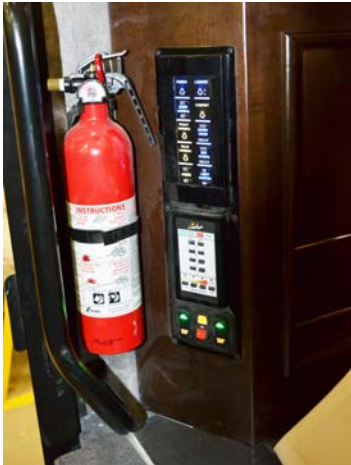
Fire Extinguisher (Located near entrance door) -Typical installation shown
