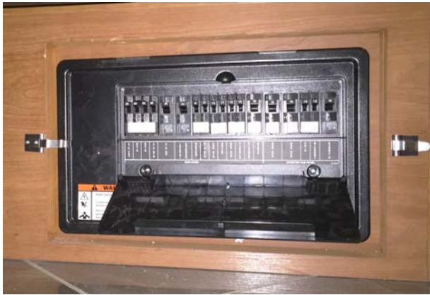
House Circuit Breakers -Typical Installation
