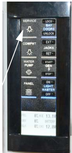
(Located in water service center) - Typical View
