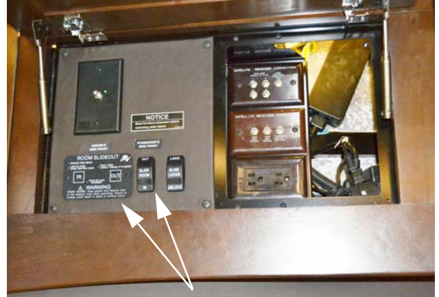
Front Slideout Switches (Located inside entrance door overhead cabinet)
