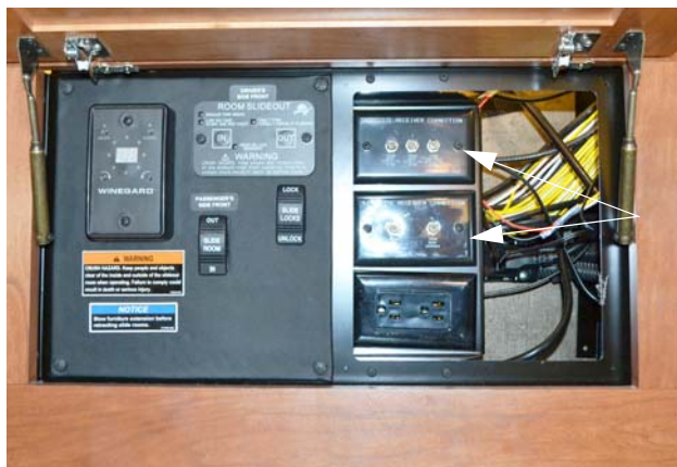
Interior Connections for Satellite Dish (Located in the overhead compartment above entrance door)
