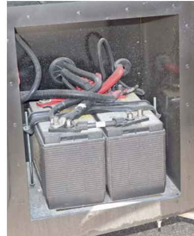
Chassis Batteries (Located behind a rear passenger side exterior door) -Typical View
