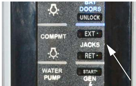
Auto Level Remote Switch (Located near entrance door and/or inside exterior service center) -Typical View
