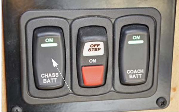
Chassis Battery Disconnect Switch (Located near entrance door) -Typical View
