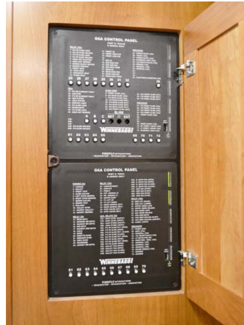
House Circuit Breakers -Typical View
