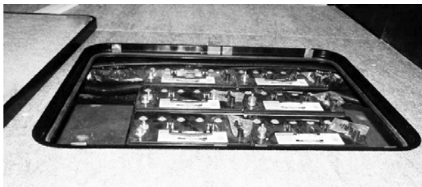
House/Coach Batteries (Shown with access cover removed) -Typical View
