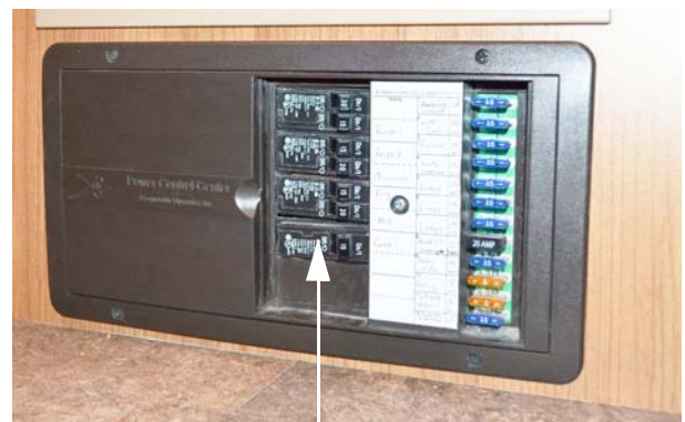
120-Volt Circuit Breakers -Typical View
