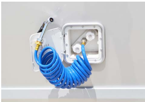
Exterior Shower/Wash Station (Typical)
