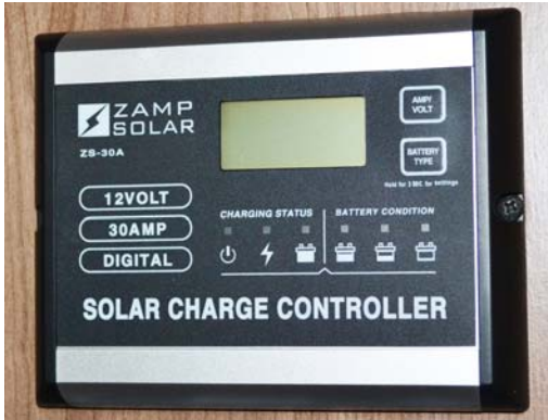
Solar Charge Controller (Located near monitor panel)
