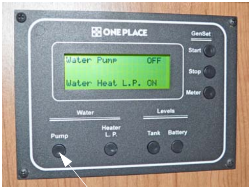
Water Pump Switch
