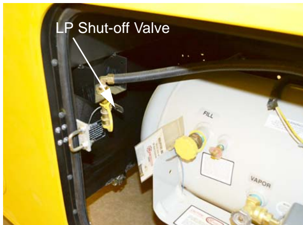
LP Accessory Connection • Model 26A - Located behind LP Tank access door on passenger side of coach
