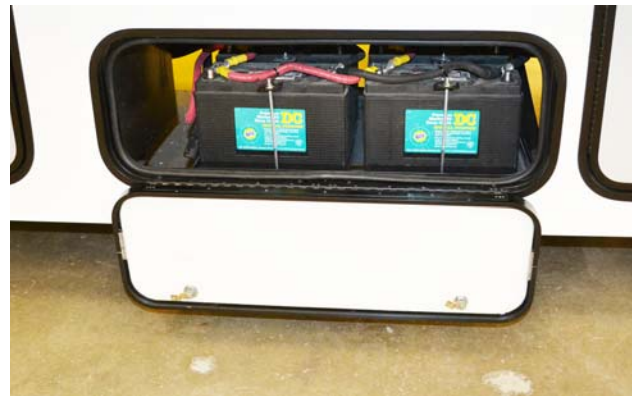
House Batteries (located behind a driver side exterior door) *Model 31C shown
