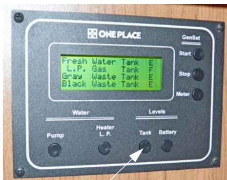
Tank Levels Switch
