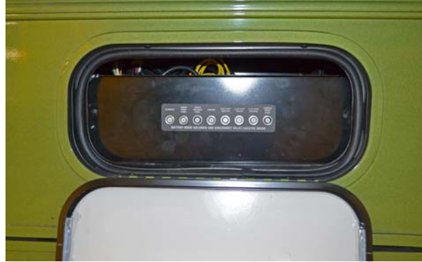
Automotive Chassis and House 12-Volt Circuit Breakers (Located inside a driver side compartment) -Typical View
