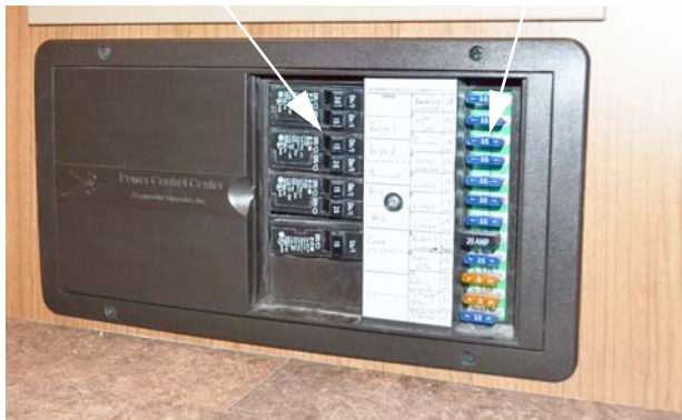
Power Center (Converter) -Typical View
