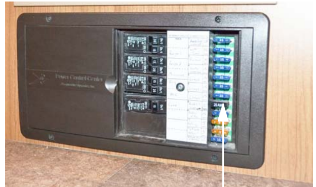
House 12-Volt Fuses (Located on right-hand side of Power Converter) -Typical View
