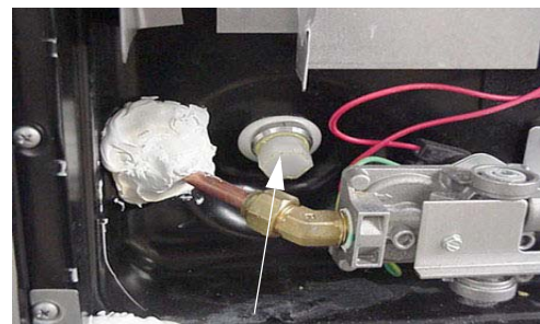
Water Heater Drain Plug (Remove with socket)
