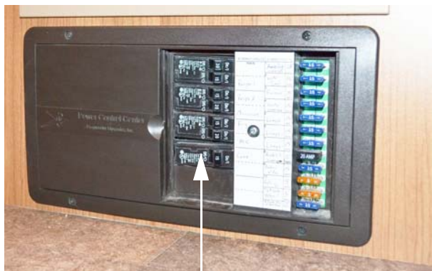
120-Volt Circuit Breakers -Typical View
