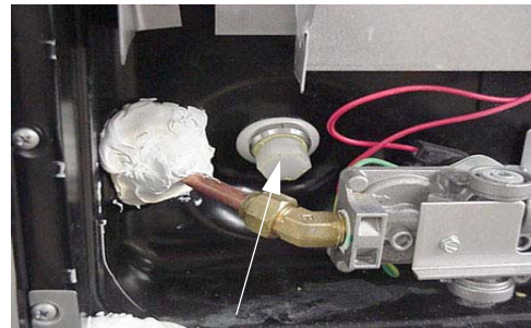
Water Heater Drain Plug (Remove with socket)
