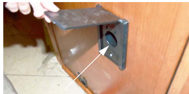
Interior Hose Outlet
