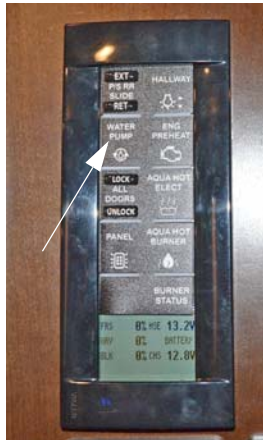
Water Pump Switch (Located on OnePlace cabinet and exterior water service center)
