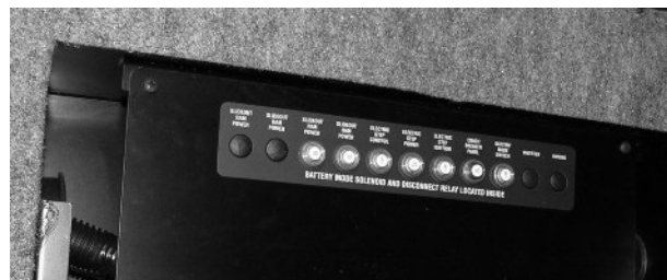
Chassis and House 12V Breakers (Located in passenger side compartment) -Typical View
