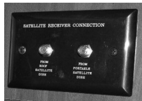
Interior Connection for Satellite Dishes (Located in cabinet near TV)
