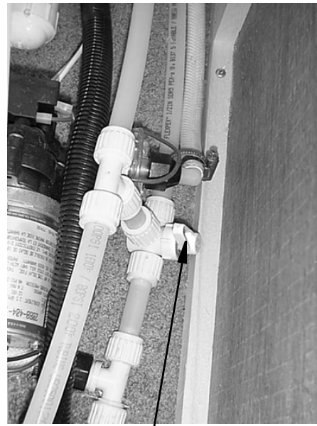
Waterline Drain Valve (Typical)
