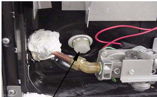
Water Heater Drain Plug (Remove with socket)
