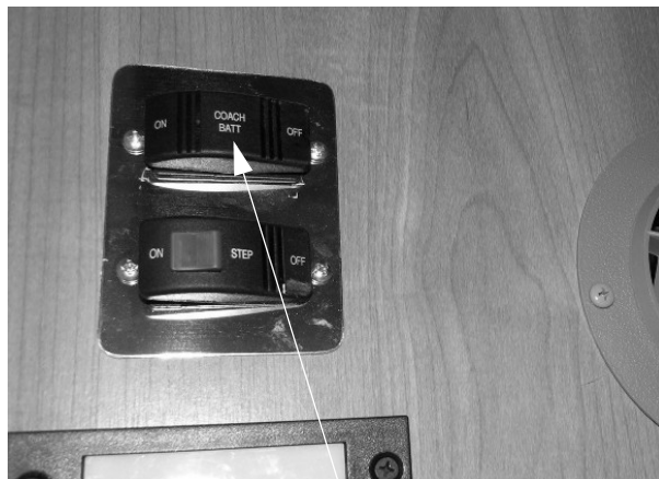
House/Coach Batt Disconnect Switch (Located near entrance door or end of galley, depending on model) -Typical View
