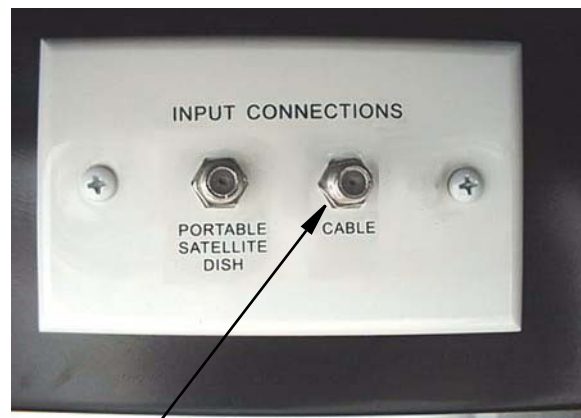
Cable TV Input Hook-Up in Utility Compartment or Shoreline Compartment depending on model
