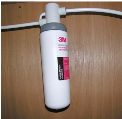
Water Filter Assembly (below Galley Sink)
