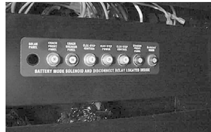
Chassis and House 12V Breakers (cover off)
