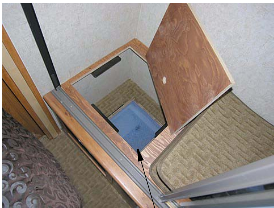
AC/Furnace Filter under wardrobe floor panel
