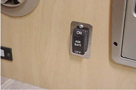
Aux. Batt. Switch - typical (Near entrance door)
