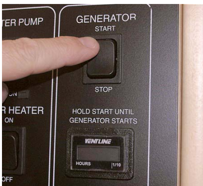
Generator Switch and Hourmeter
