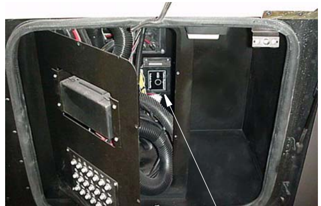
Keyless Entry Control Box in 12-volt electrical compartment.
