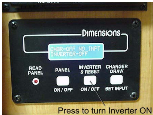
Inverter/Charger Control Panel
