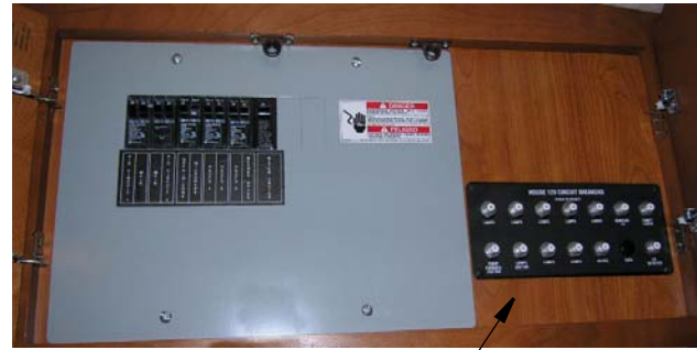
House 12-Volt Circuit Breaker Panel
