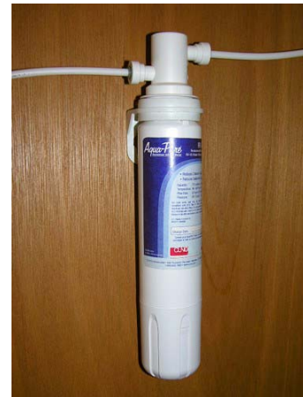
Water Filter Assembly below Galley Sink
