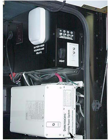
Inverter Charger Unit Location in utility compartment
