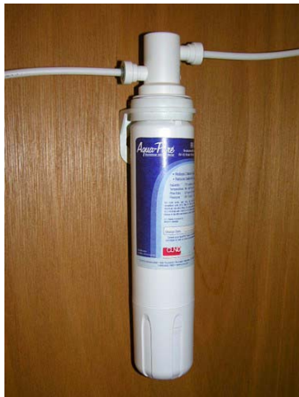
Water Filter Assembly below Galley Sink
