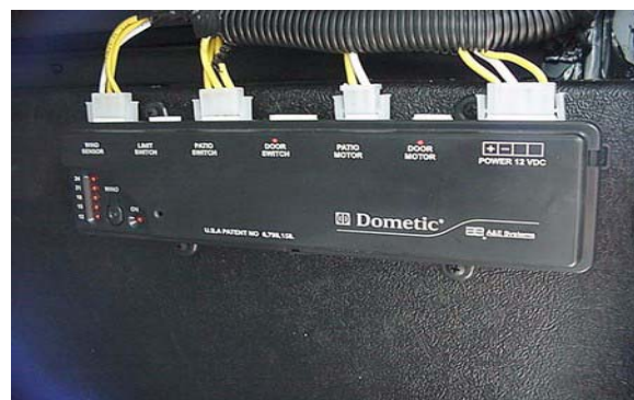
Awning Control Box (located in exterior compartment)
