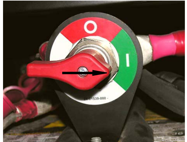
Diesel Chassis Battery Cutoff Switch (inside battery storage compartment)
