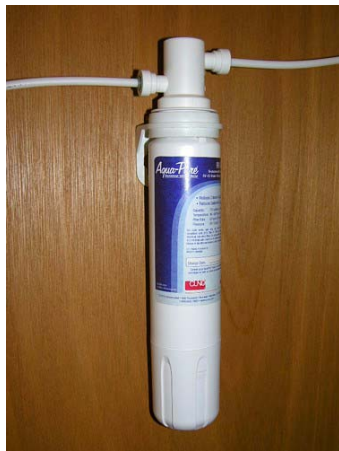
Water Filter Assembly (Located below galley sink)
