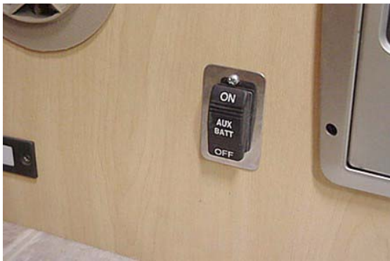
Aux. Batt. Switch - typical (Near entrance door)
