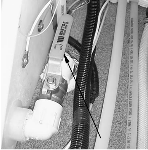
Water Tank Drain Valve (Typical)
