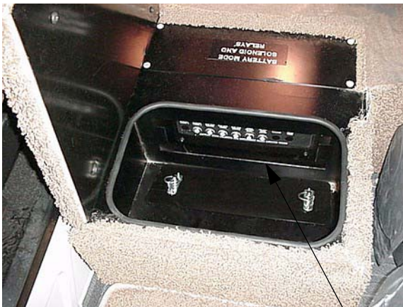
Chassis/House 12V Circuit Breakers behind cover panel in floor compartment between front seats.
