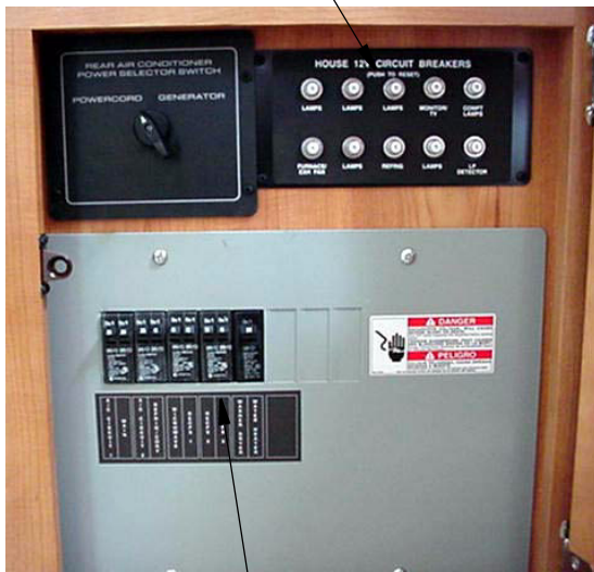
110-Volt Circuit Breakers
