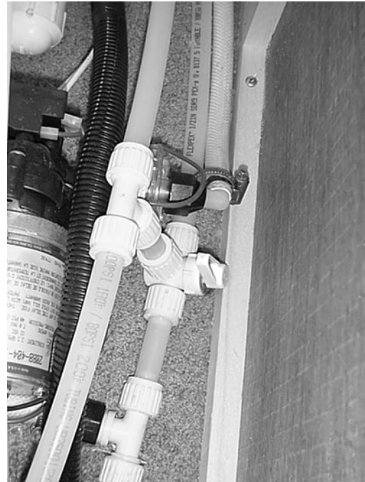
Water Heater By-Pass Valve (Typical)
