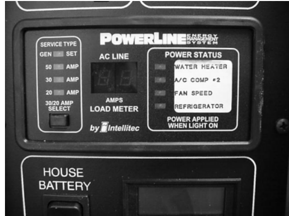
EMS Display on Monitor Panel
