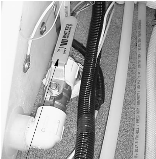
Water Tank Drain Valve (Typical)
