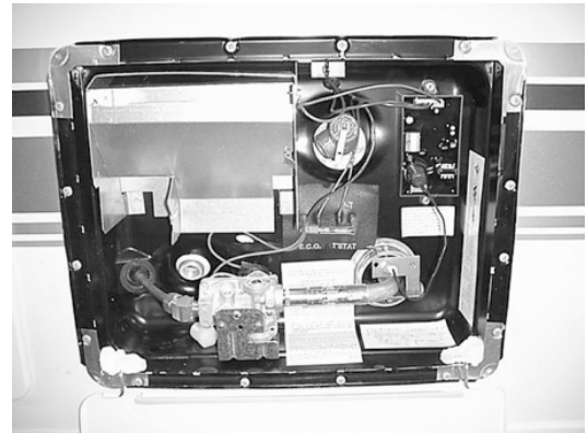
Water Heater Exterior Service Access
