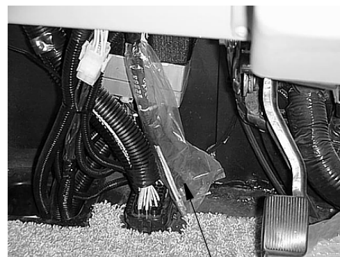
CB Power Wires (in plastic sheath)
