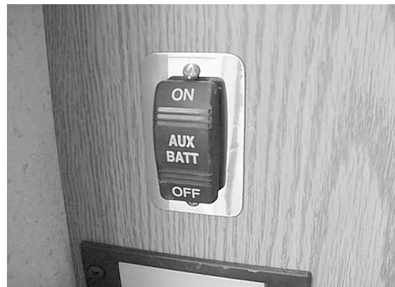
Aux. Batt. Switch (Near entrance door)
