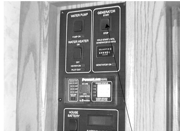
Generator Switch and Hourmeter
