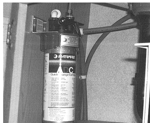
Water Filter Assembly - Below Galley Sink
