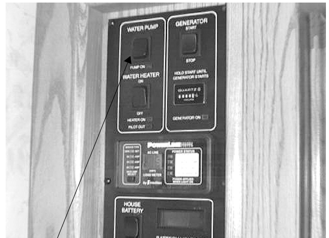
Water Pump Switch
