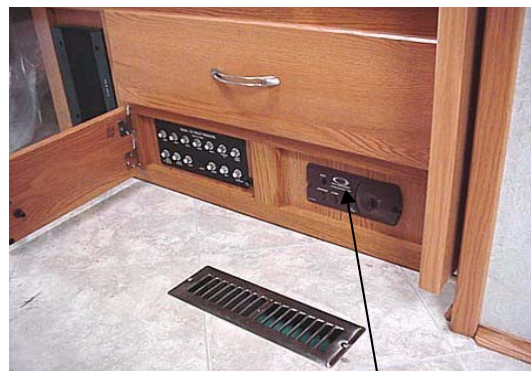
LP Gas Alarm
