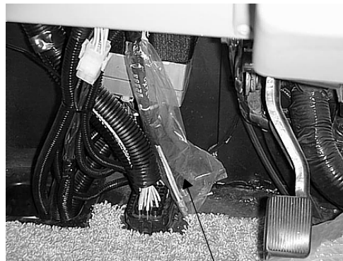
CB Wires (in plastic sheath)
