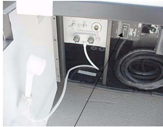
Inverter Charger Unit Location in shoreline compartment
