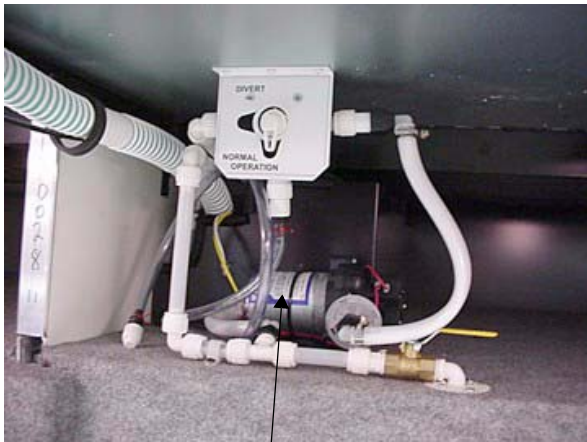
Water Pump (typical)
