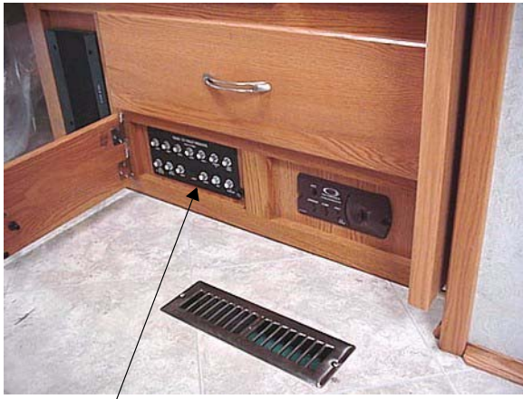
House 12-Volt Circuit Breaker Panel
