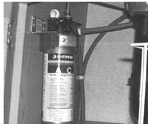
Water Filter Assembly - Below Galley Sink
