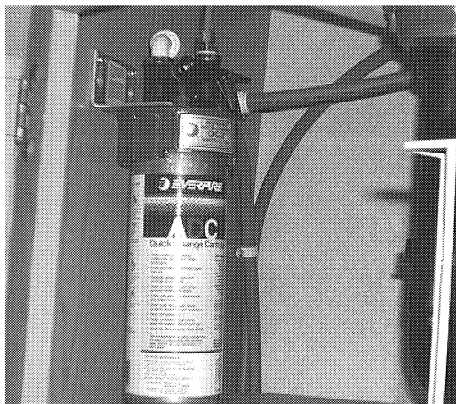
Water Filter Assembly - Below Galley Sink
