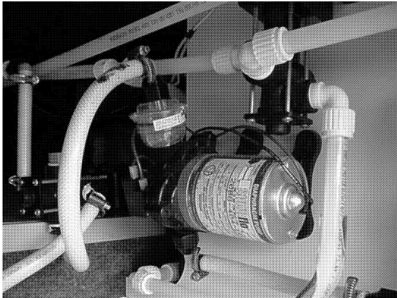
Water Pump and Filter
