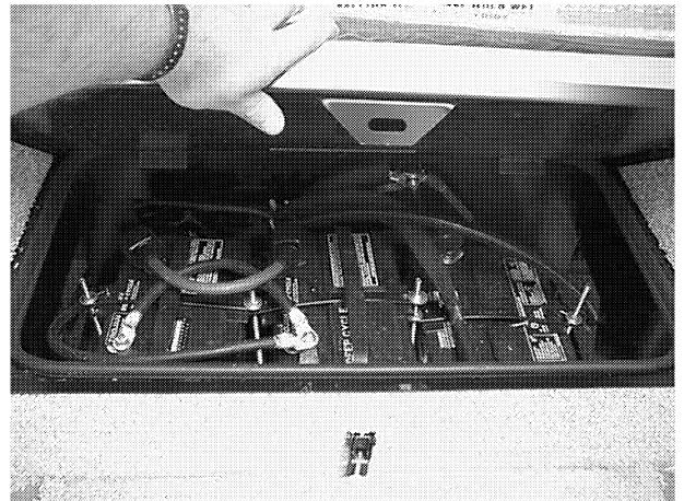
Lift step to access batteries
