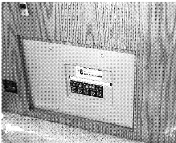
House 110-volt Breaker Panel
