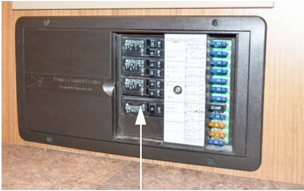
120-Volt Circuit Breakers -Typical View
