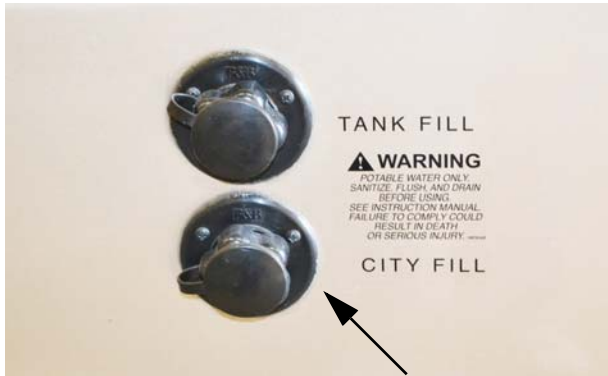
City Fill Inlet (Located on the left sidewall)
