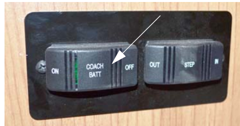
House/Coach Battery Disconnect Switch (Located on front side of galley)
