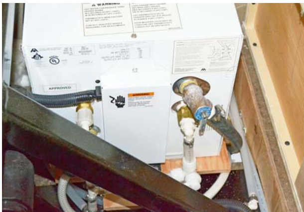
Water Heater Interior Service Access (located below forward facing dinette seat) -Typical View
