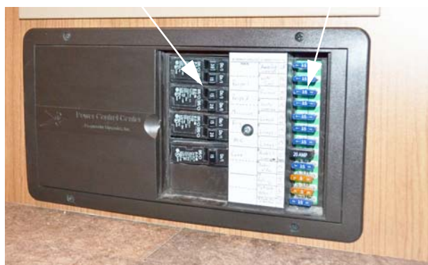
Power Center (Converter) -Typical View
