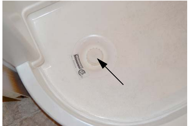
Shower Drain Strainer (Located in shower floor) -Typical View
