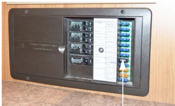
House 12-Volt Fuses (Located on right-hand side of Power Converter) -Typical View
