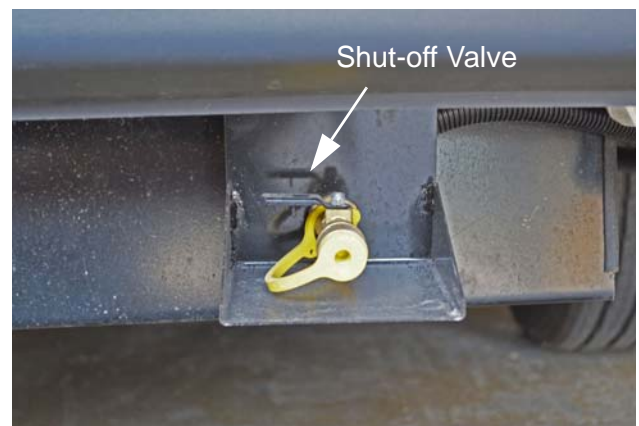
LP Accessory Connection (Located at rear of coach) -Typical View
