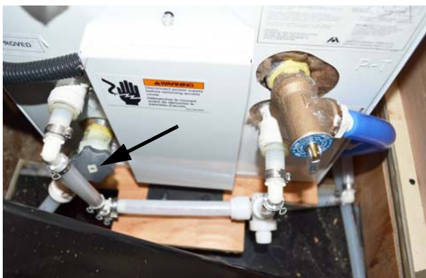
Water Heater Drain Plug
