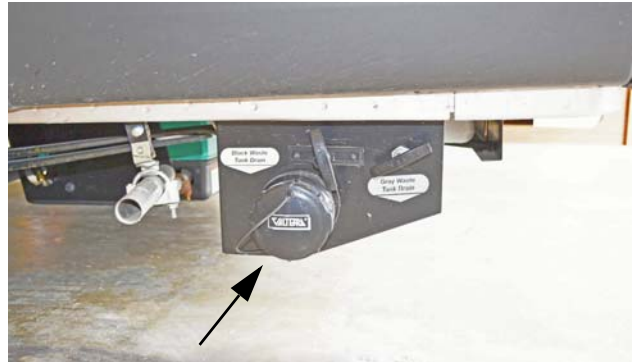
Sewage Drain Outlet (Located beneath coach) -Typical View
