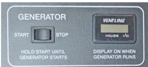
Generator Switch and Hourmeter on monitor panel
