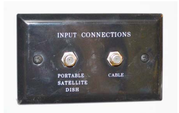
Exterior Connection for Satellite Dish and Cable TV (Located in utility compartment) -Typical View
