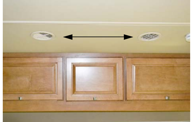
Supply/Return Air Vents (Located throughout the ceiling of the coach) -Typical View
