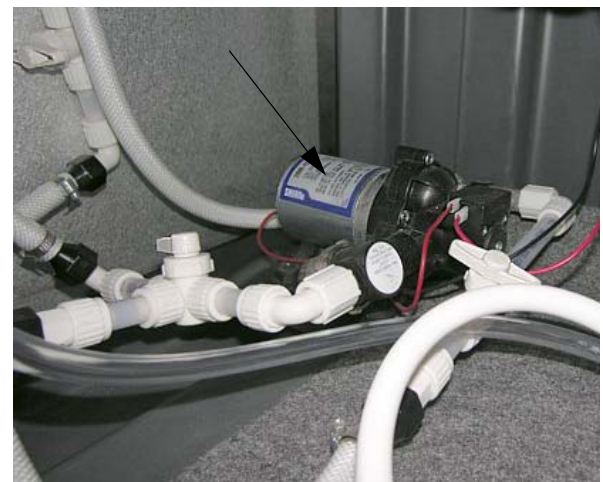
Water Pump -Typical View
