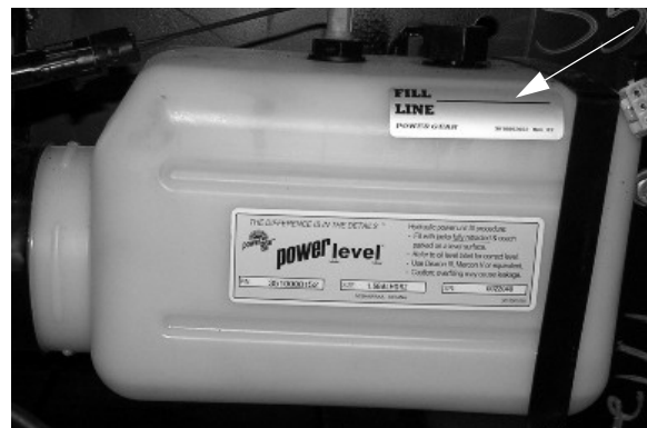
Hydraulic Oil Reservoir (Located underneath front entry step) -Typical View
