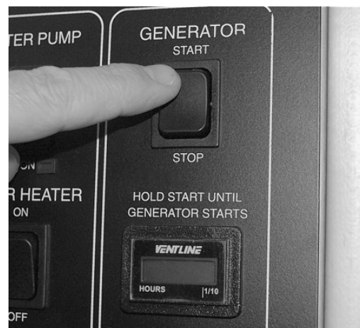
Generator Switch and Hourmeter (Located on monitor panel) -Typical View
