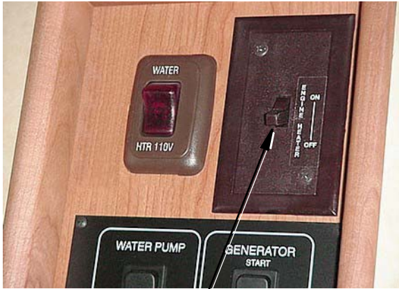
Diesel Engine Heater Switch -Typical View
