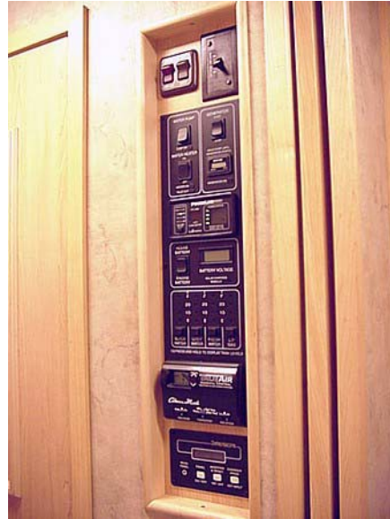
OnePlace Monitor Panel -Typical View
