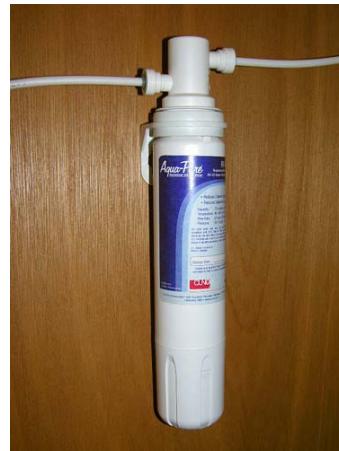
Water Filter Assembly (Located below galley sink)
