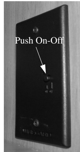
TV Signal Amplifier Power Switch -Typical View
