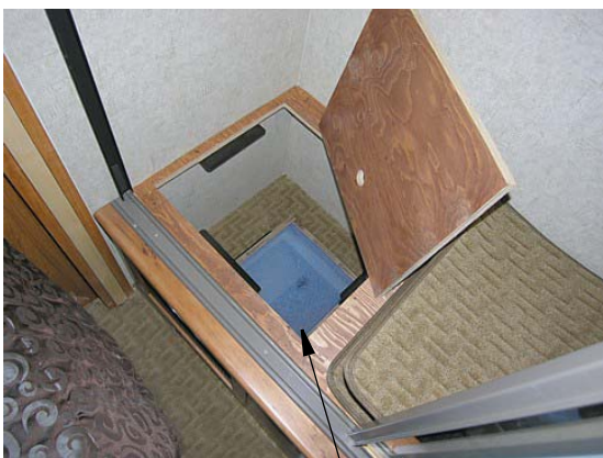
AC/Furnace Filter under wardrobe floor panel
