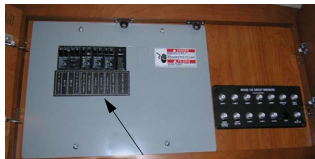
House 120-Volt AC Circuit Breaker Panel
