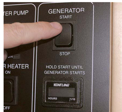
Generator Switch and Hourmeter
