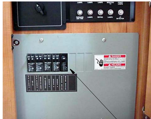
120-Volt House Circuit Breakers
