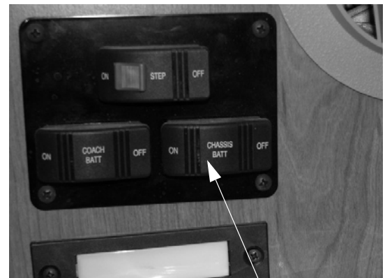
Chassis Battery Disconnect Switch * Model D31E shown (Located inside the entrance door)
