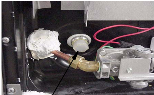
Water Heater Drain Plug (Remove with socket)
