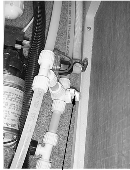
Waterline Drain Valve (Typical)
