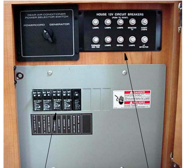
120-Volt House Circuit Breakers
