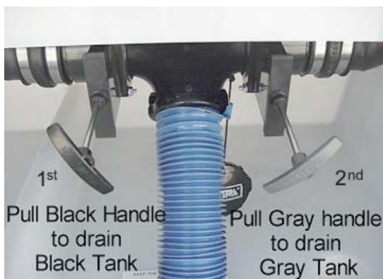
Holding Tank Dump Valves -Typical View
