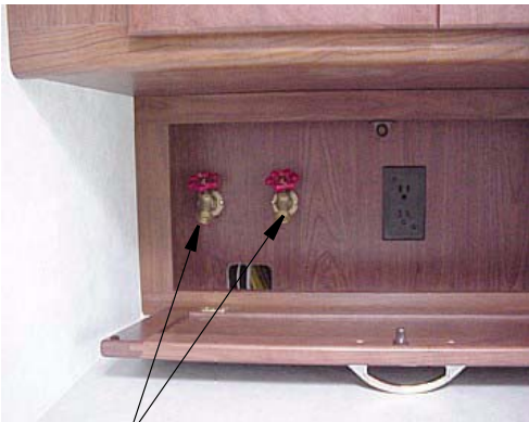
Water Supply Faucets - Typical
