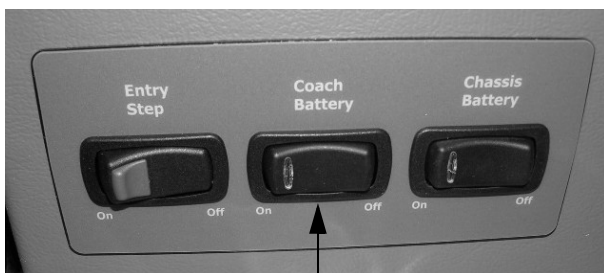
Aux. Battery Disconnect Switch (Near Entrance Door)
