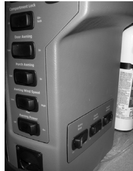
Awning Control Switches - Typical View (Located near entrance door)
