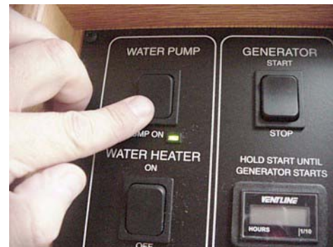
Water Pump Switch on OnePlace Panel
