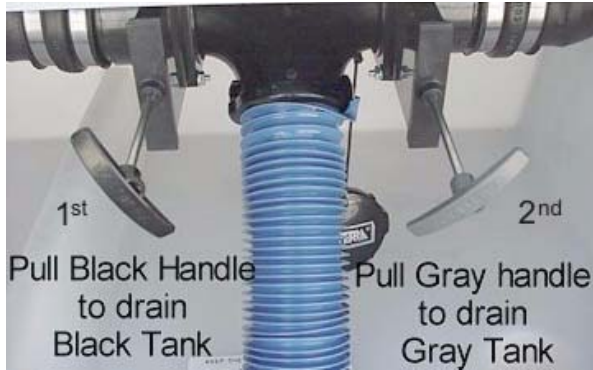
Holding Tank Valves (Typical)
