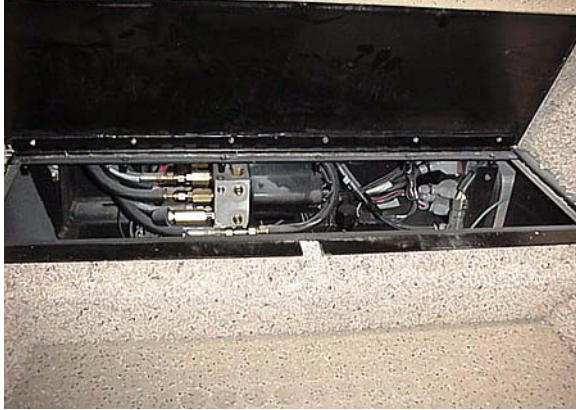
Hydraulic Pump beneath Entry Step
